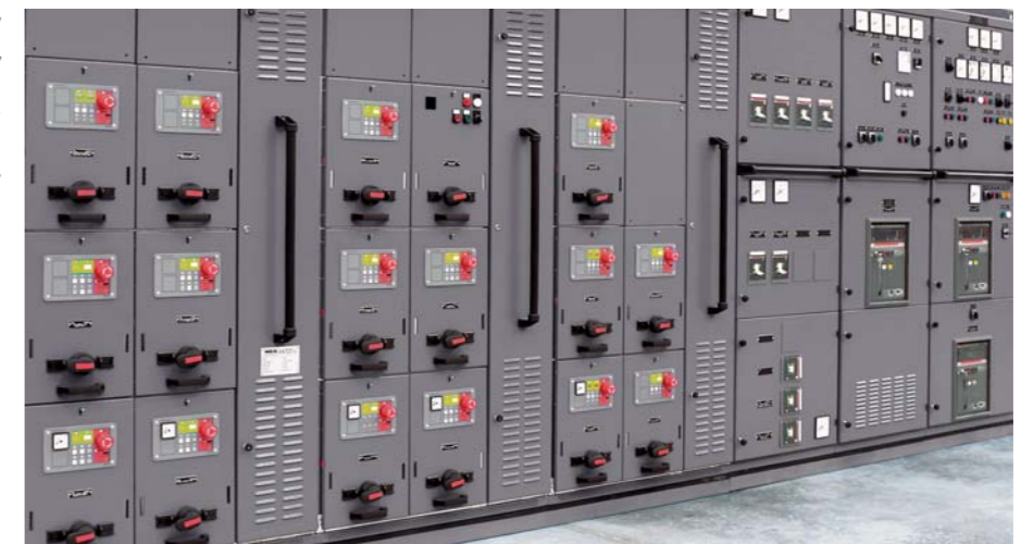
Power Motor Control Center 690V-3000A-40kA Fincantieri RO-RO Passenger Vessel - Finn Lines
