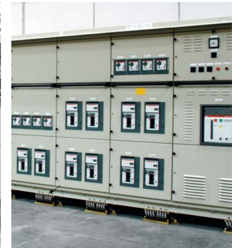
Main Distribution Switchboard 660V-4000A-74kA Fincantieri Aircraft carrier "Conte di Cavour"
