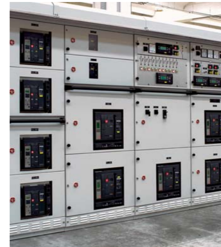
Main Switchboard 440V-5780A-75KA Fincantieri (Italy-France project) "HORIZON" Class Frigate
