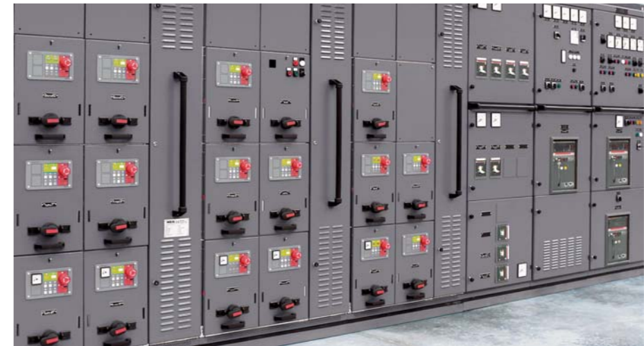
Power Motor Control Center 690V-3000A-40kA Fincantieri RO-RO Passenger Vessel - Finn Lines
